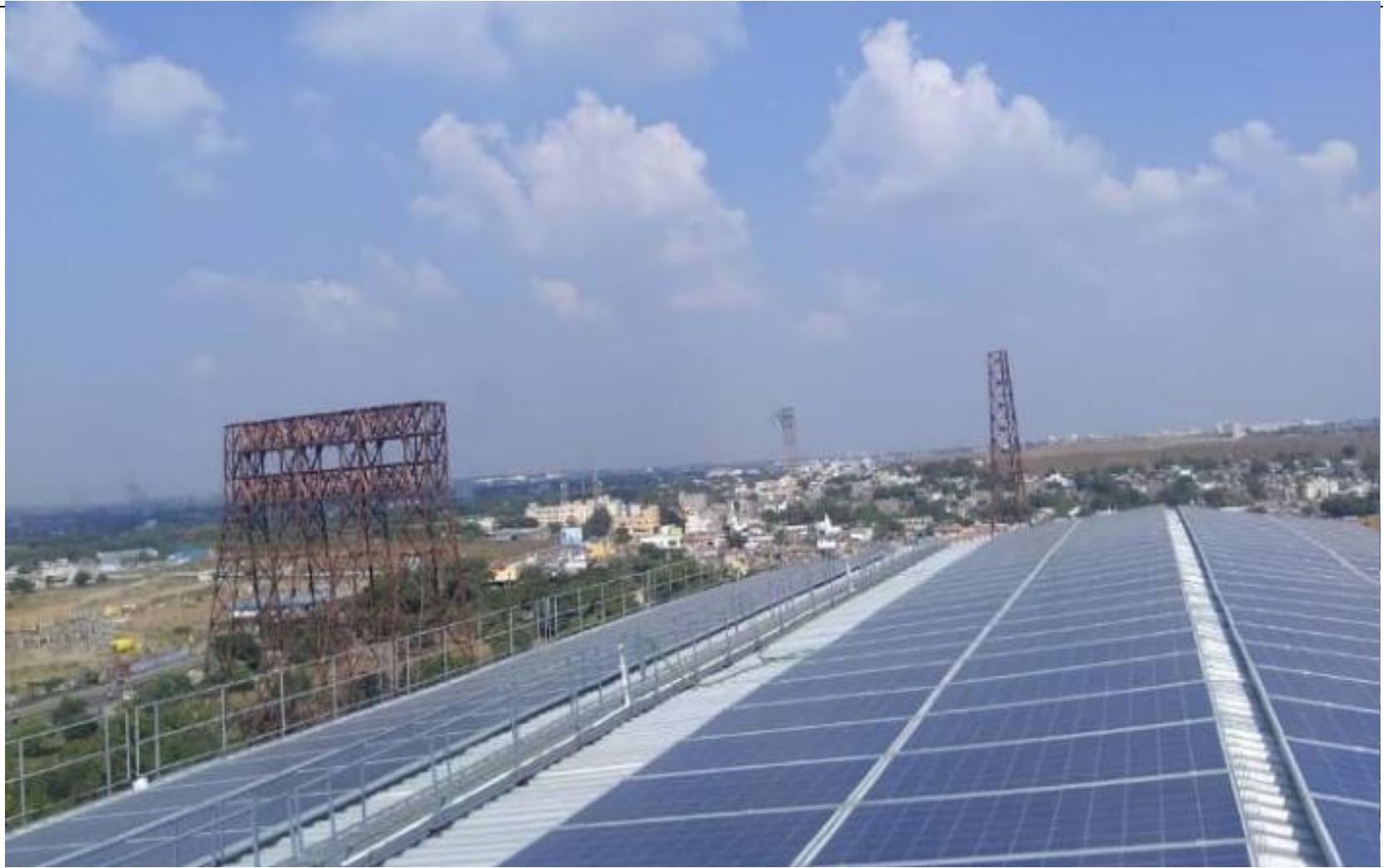
Image No. 3 : Rooftop Solar Panels Installed
