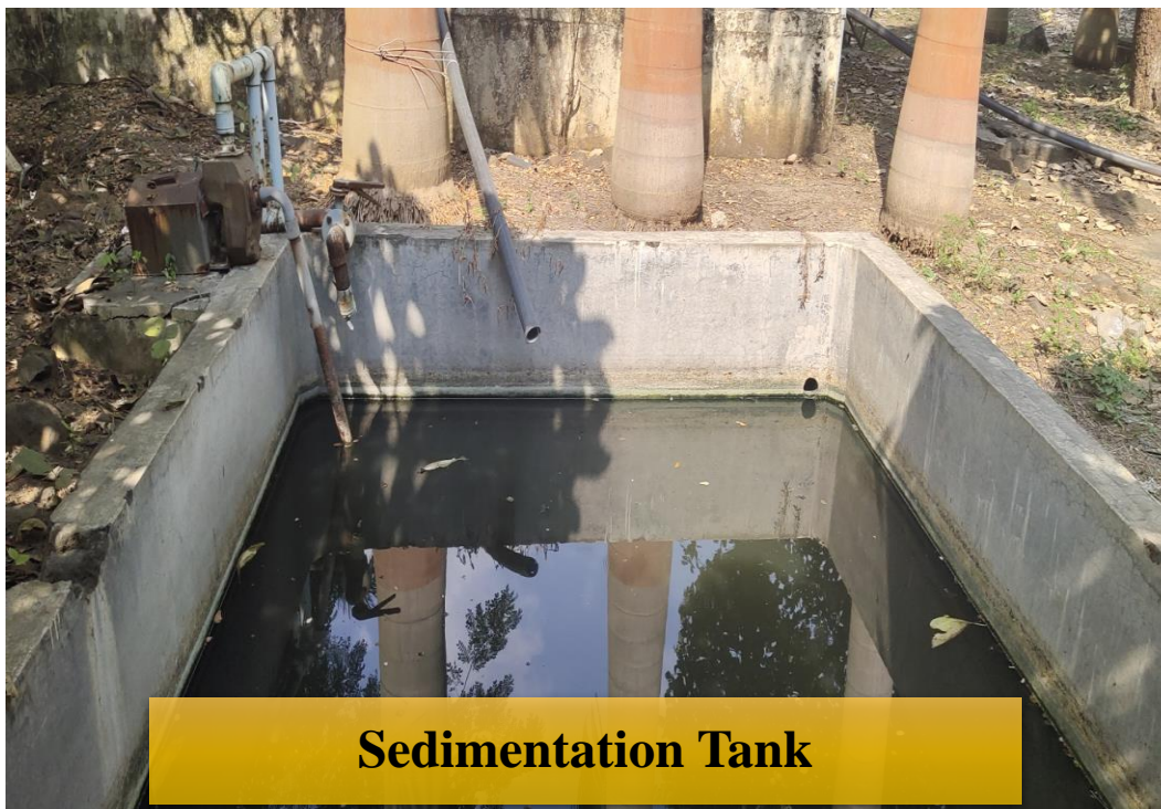
Photograph No. : Sewage Treatment Plant
