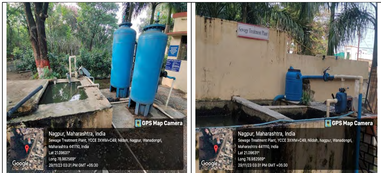
Image No. 30: STP at YCCE
