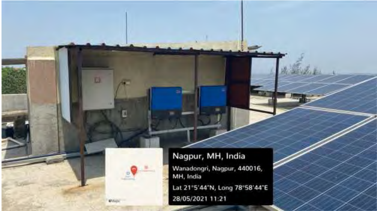
Solar Panel on Roof of Civil Building
