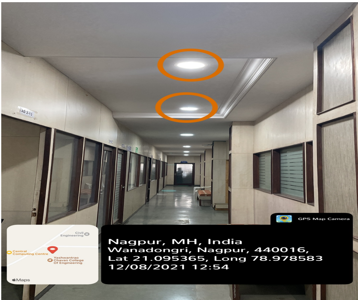
LED Lamps in Corridor
