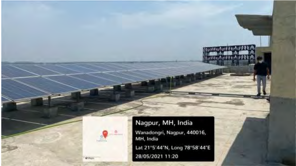
Solar Panel on Roof of Civil Building
