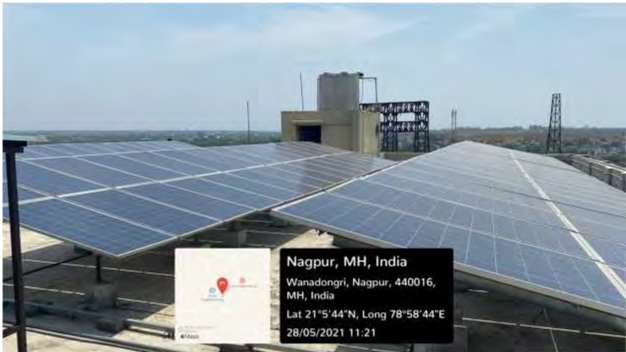
Solar Panel on Roof of Civil Building
