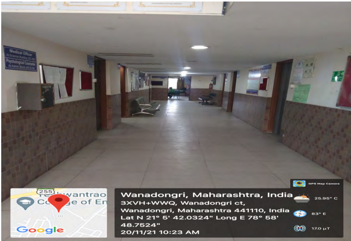
LED Lamps in Corridor
