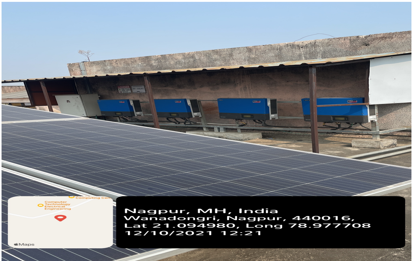
Solar Panel on Roof
