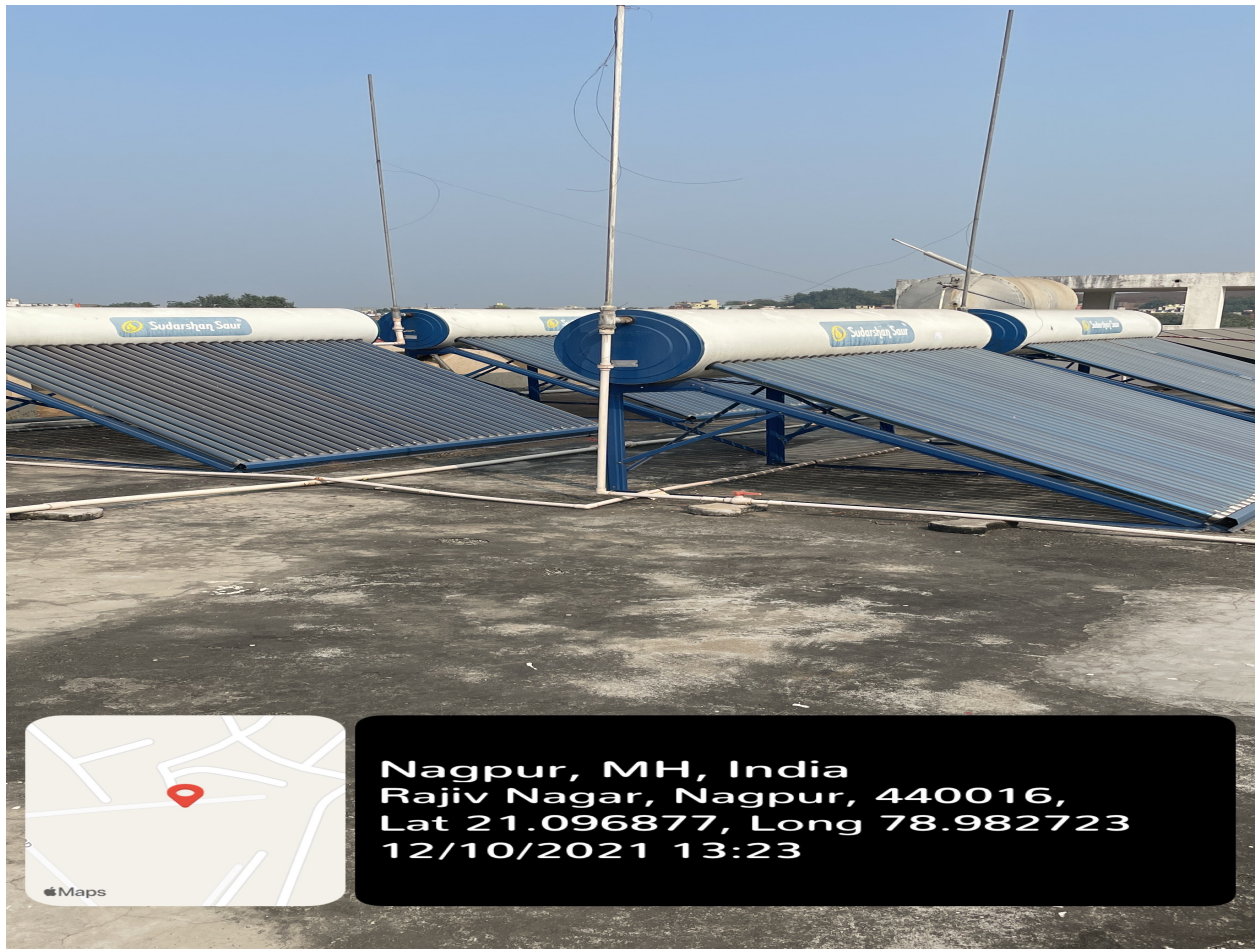
Solar Panels for Water Heating in Hostel
