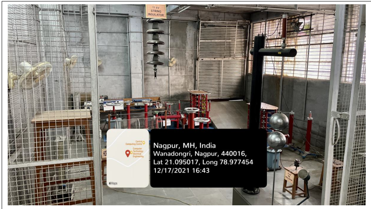
EL-0-11- High Voltage Engineering Lab
