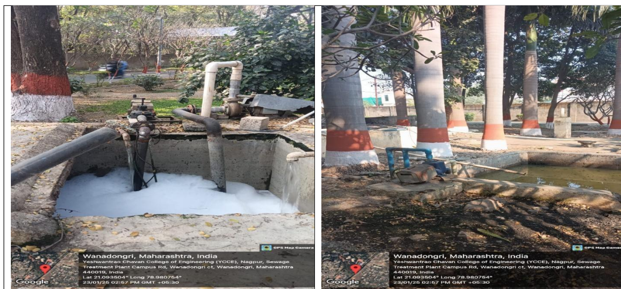
Image No. 30: STP at YCCE
